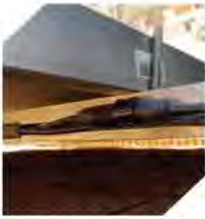
Cable Management in Rails
